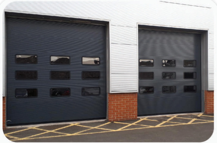
Garage Overhead Doors
