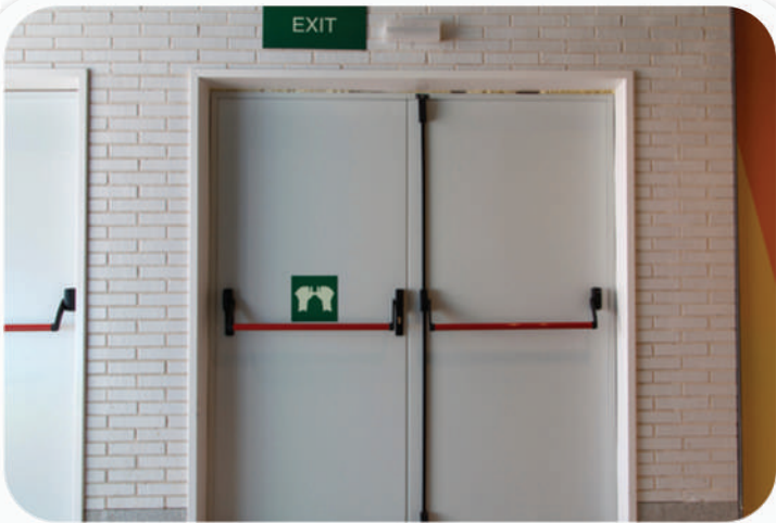
Steel Fire Doors
