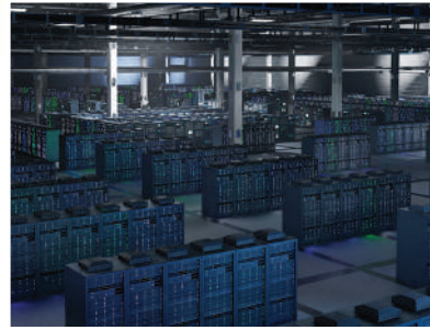
Data Centers & IT Facilities
